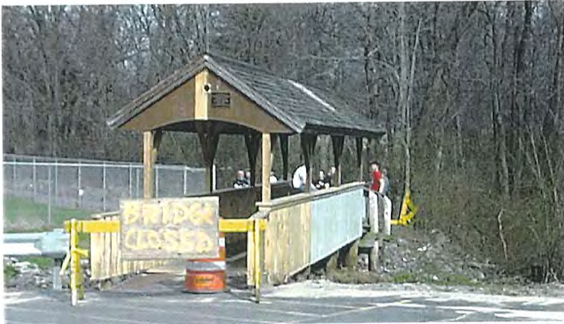
Covered Bridge over Trout Brook Tributary behind Town Offices - a Popular Hang Out Despite Recent Vehicular Damage.
