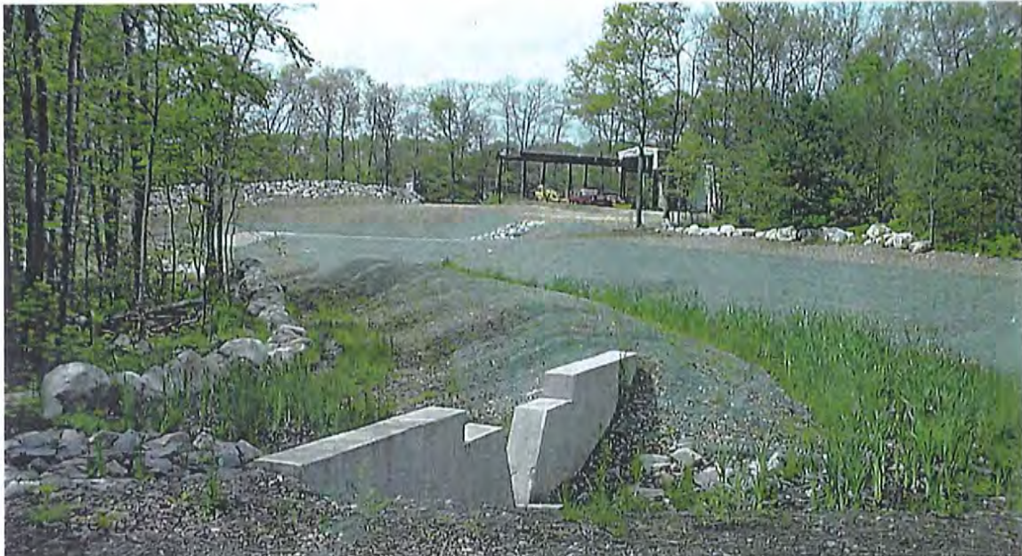
New Industrial Park Storm Water Control System - Detention Pond with Tapered Weir North of Murphy Drive
