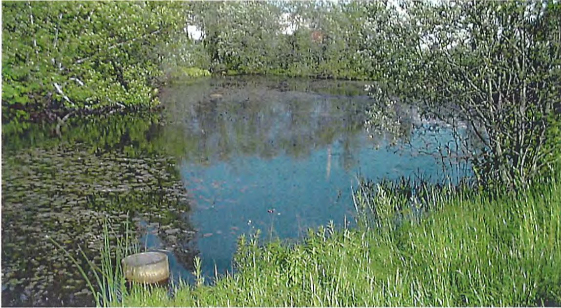
Industrial Park Storm Water Mitigation; Enhanced Detention Pond at Murphy Drive with Modified Outlet Structure in Foreground
