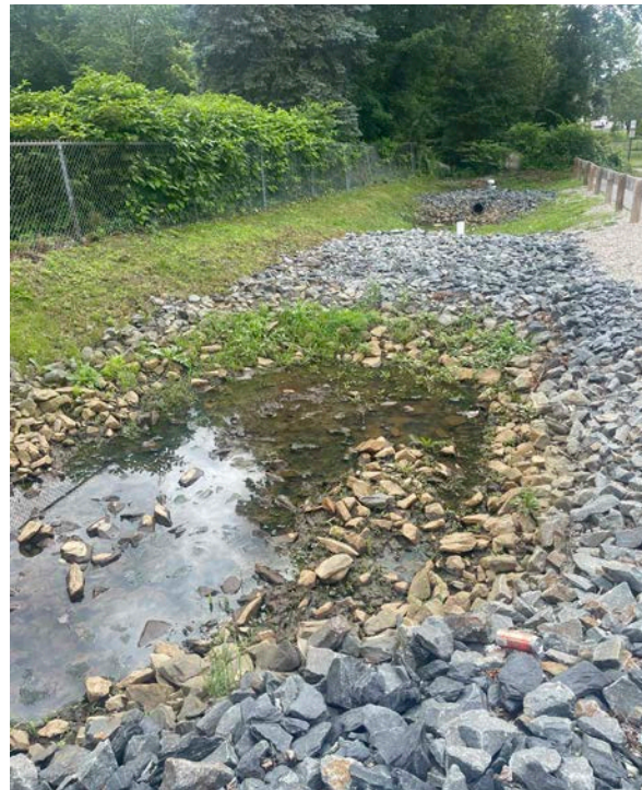
Figure 2.10. Green infrastructure at Town Hall
