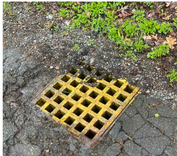
Figure 2-20. Catch basin draining to wetlands with no buffer
